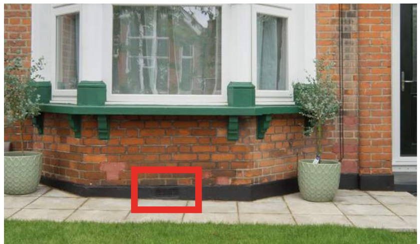
Smart air bricks located at the property
