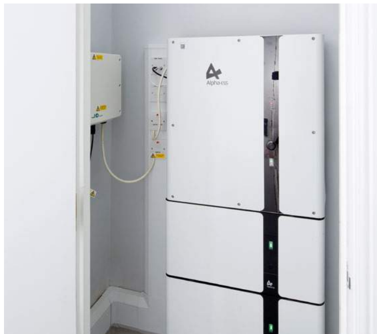
Alpha battery storage in position
